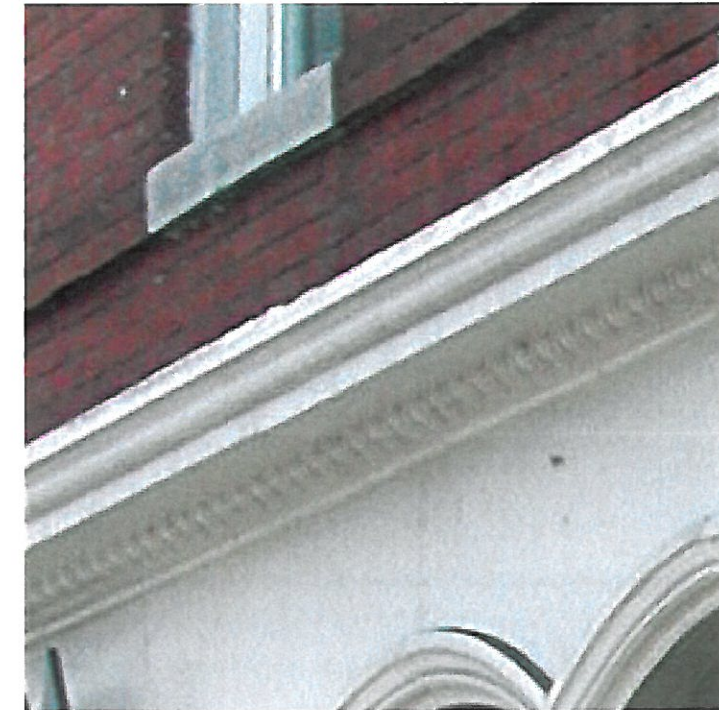
Trim separation between materials
