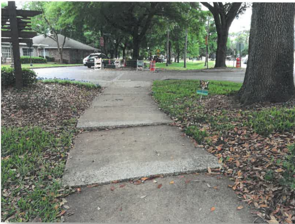
Exhibit 3 – Example of sidewalk joints with tripping hazards
